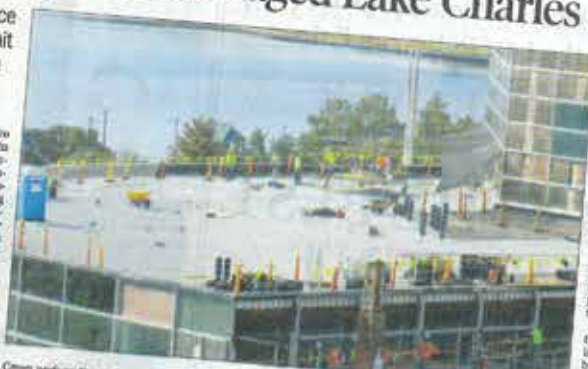
Construction work on the roof and facade of the Capital One Tower in downtown Lake Charles on Wednesday. STAFF PHOTO BY ALIEN MASCHKE
